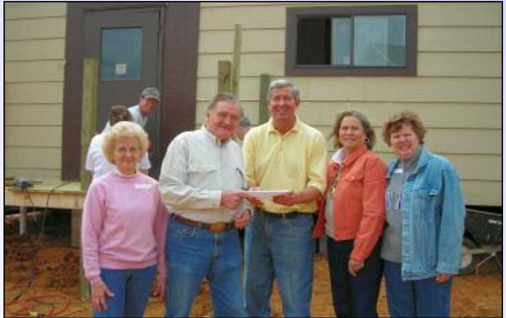
Bill and Al Langford, Danny Berry, Kay Foshee, and Pam Langford .....FBC Missions Men building porch and steps in background
